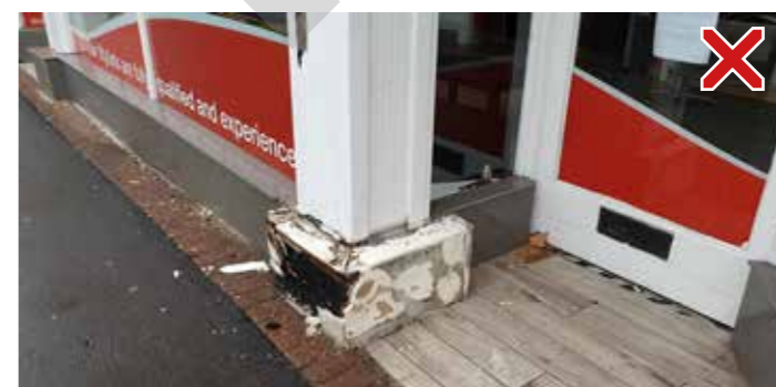
Inappropriate material will decay quickly near ground level, creating undesirable appearance
