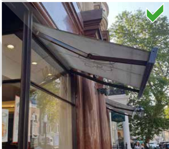
20th century metal shop front. Blind box incorporated at head of windows
