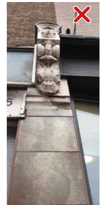
ornate corbel and capitol retained, inappropriate facing material placed on pilaster, with unsatisfactory detailing between old and new
