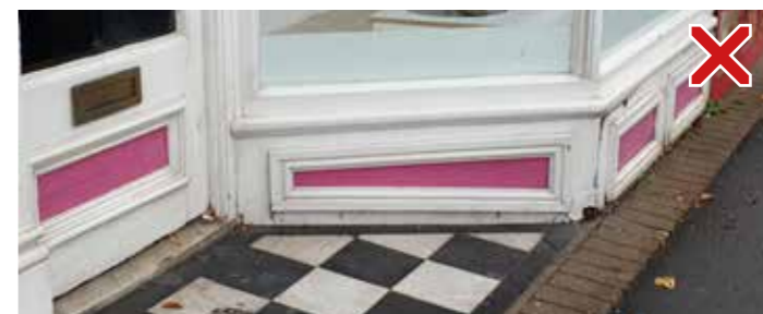
Inappropriate decoration of panelled scheme, applied as a copy of an original stall riser. Colour emphasises the difference in design detail of window frame and planted riser
