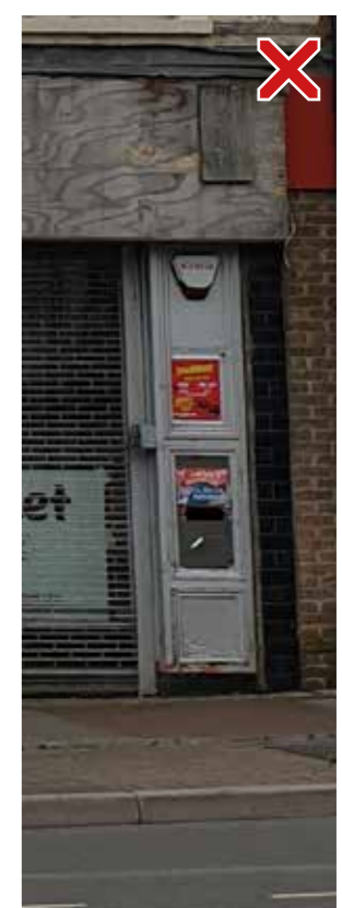
Original capitol overridden with enlarged fascia.
